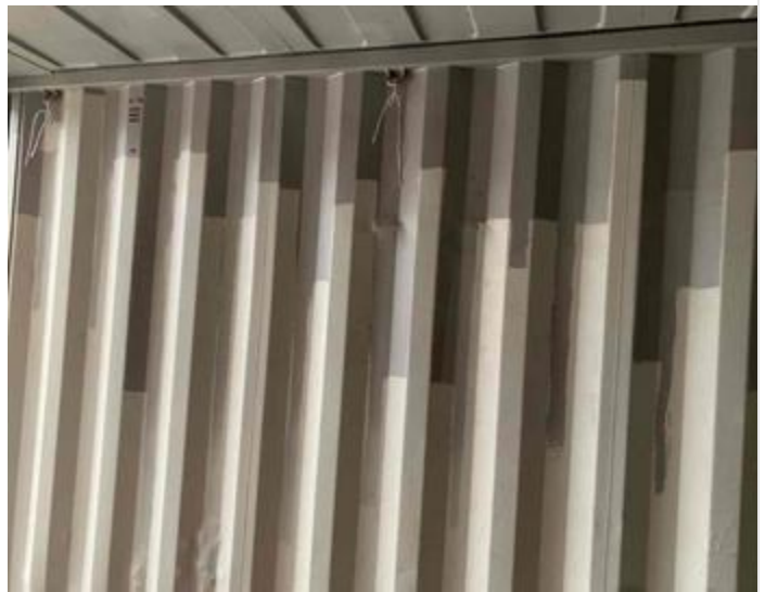
8.1.6. No defects inside container CEILING 集装箱天花板缺陷
